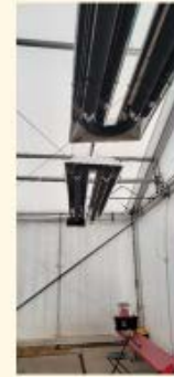
Radiant Heaters Above Deck
