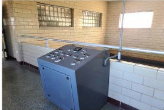
DUAL-MEDIA FILTER CONTROL CONSOLE
