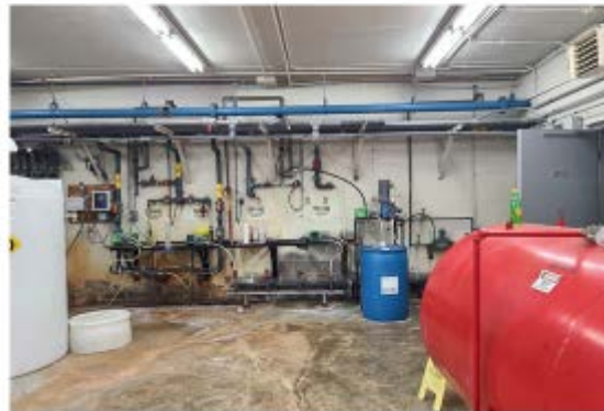
CHEMICAL FEED ROOM
