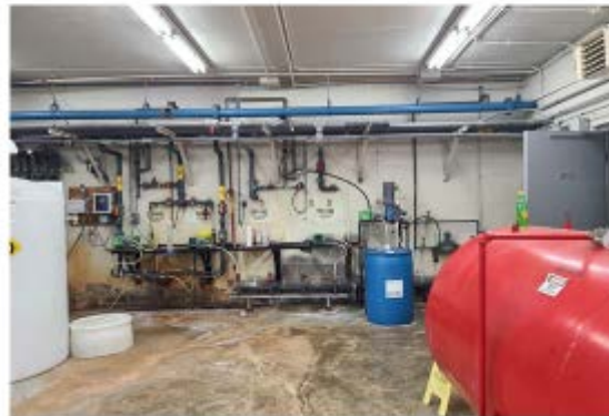
CHEMICAL FEED ROOM
