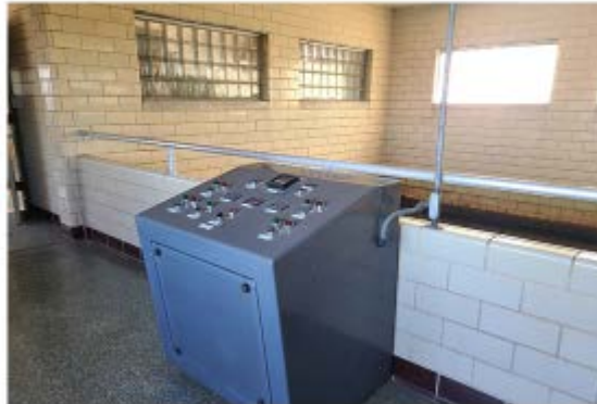
DUAL-MEDIA FILTER CONTROL CONSOLE
