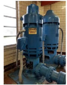
Water Treatment Plant Motor Control Centers – High Service Pump Replacement
