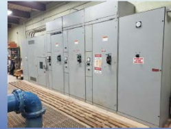
Motor Control Center: Located in finish pump house
